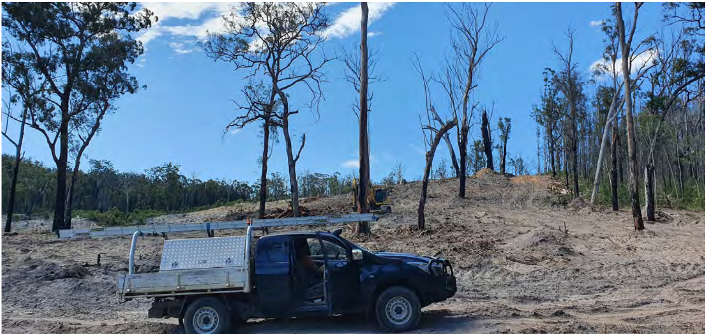
Plate 1-2. Retained habitat trees subject to staged clearing as part of quarry expansion works.
